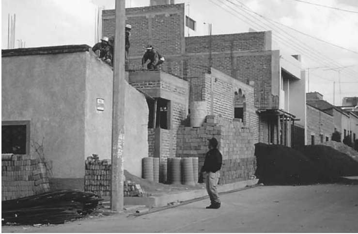
Photograph 2.5. Construction Site in Degollado. Piles of rebar, stacks of bricks, cement pipes, and heaps of gravel—as well as a two-story house such as the one rising in the background—show how migration is transforming the appearance of small towns throughout Mexico.
