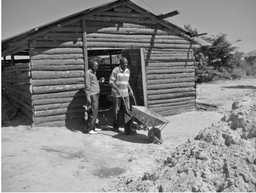
FIGURE 2. Pouring cement for the floor of the Freedom Bible Church chapel in 2013 with Pastor Ephraim and Mr. Moyo, the church administrator.
